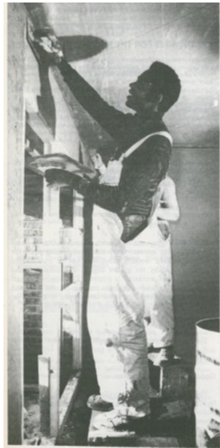
DLOs provide facilities for proper training, and help create conditions where planned job training programmes can become a reality. Above: a training display given by GLC direct labour force, 1976. Picture: GLC.
